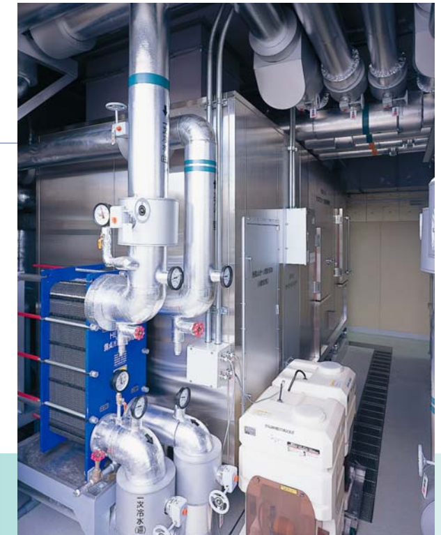
Equipment around the air-processing unit
