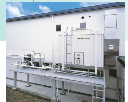
Deodorizing unit and Cooling tower
